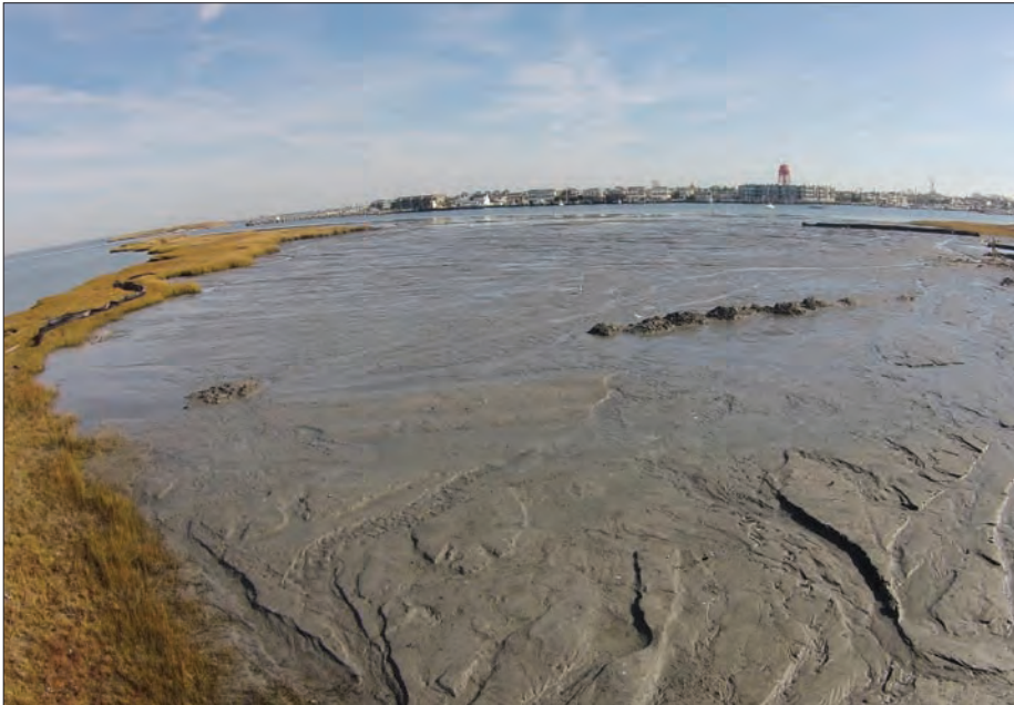
A dredging and marsh restoration demonstration project on Mordecai Island near Long Beach Island, N.J., is using dredged material from a shoal in the New Jersey Intracoastal Waterway to restore the eroded area and elevate the adjacent marsh. Planting of the restored area will be done in spring 2016.
