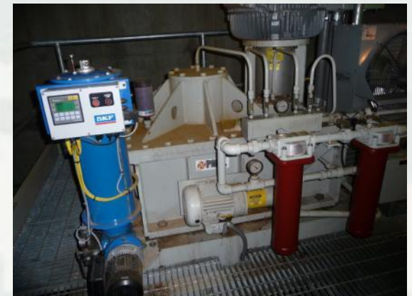
Grease metering system
