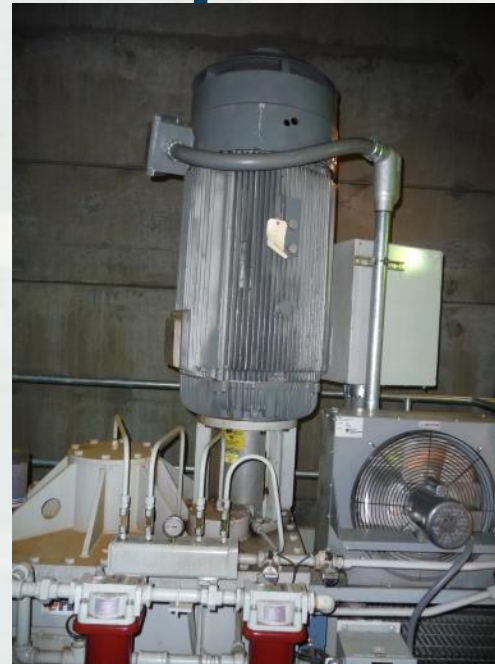
Fish pump at John Day dam.
