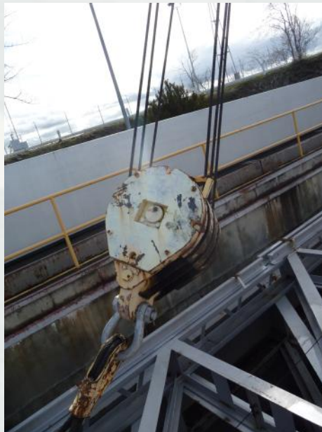
Large crane & hoist at the John Day Dam
