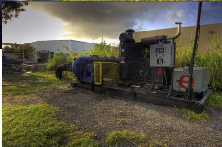
Booster Pump Placed in Industrially Zoned Area
