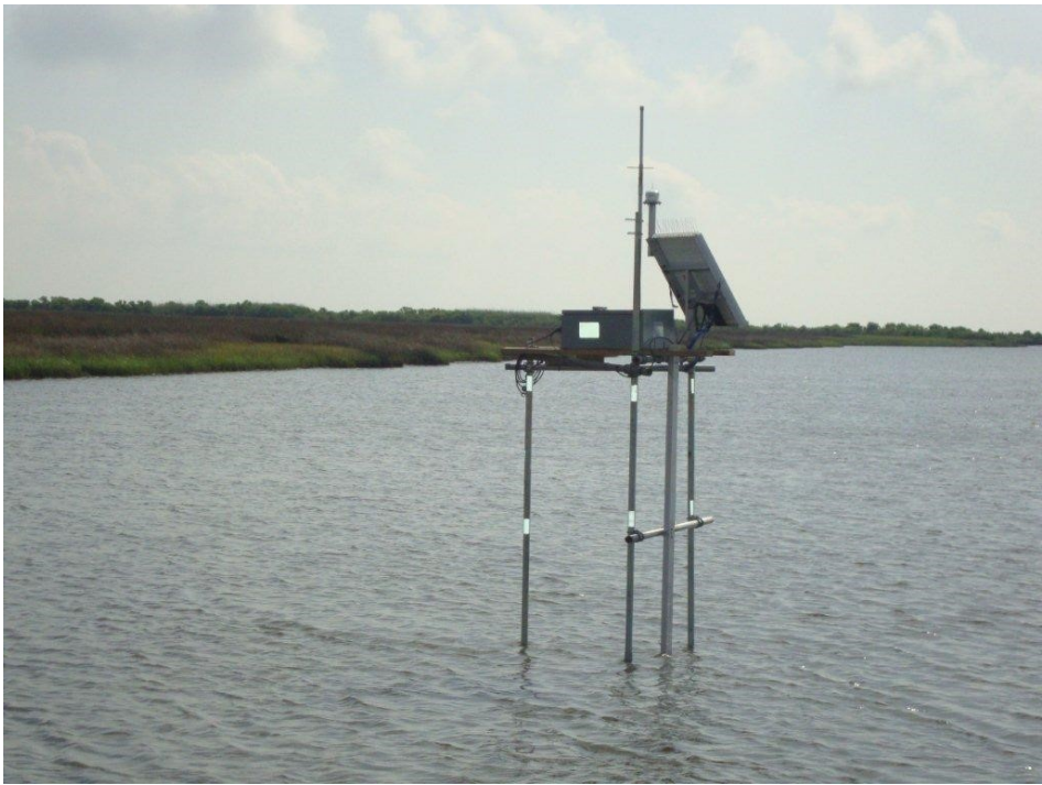
Figure 4. Image of the ADV platform type to be installed by USACE staff.
