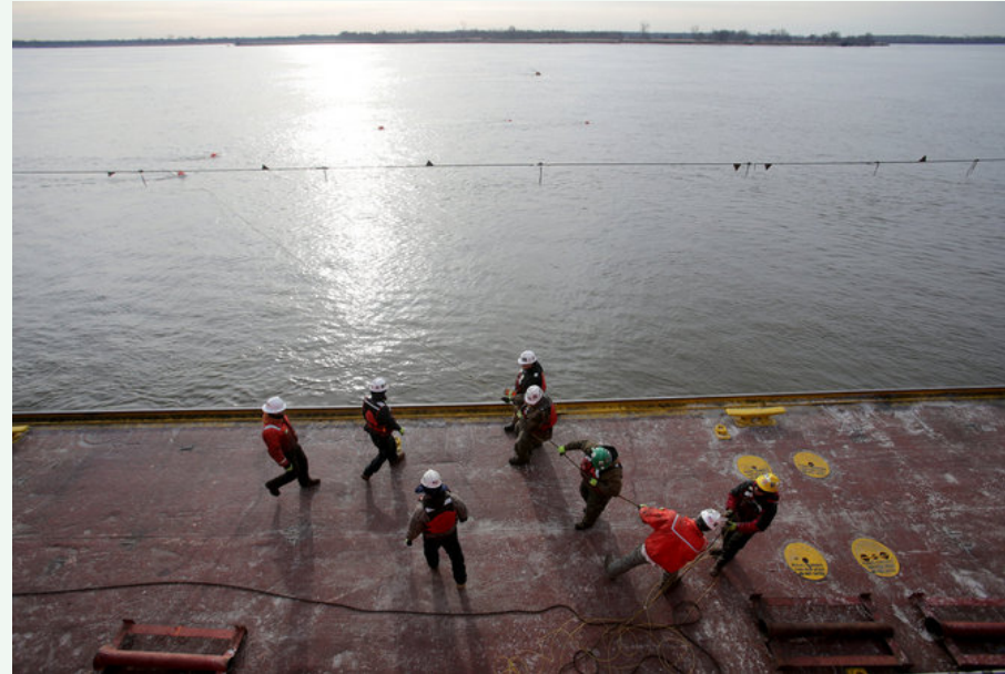
Downlines that are connected to explosives are pulled from the water by workers aboard the drillboat Apache after a morning blast off Chester, Pa., as part of the Army Corps' Delaware River deepening project, Wednesday, Jan. 20, 2016. (Tim Hawk | For NJ.com)
