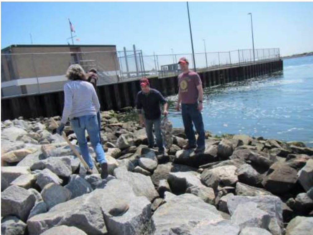
Philadelphia District engineers and biologists placing oyster shells in crevices of existing revetment during EWN demo workshop in Rehoboth Beach, DE.
