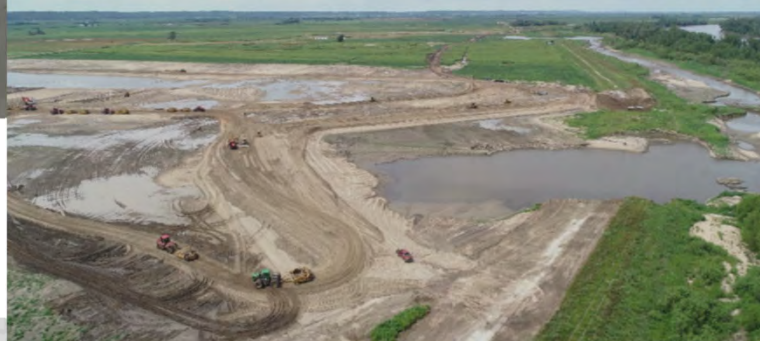
F Breach, July 2020 (with temp ring levee to prevent site from flooding)
