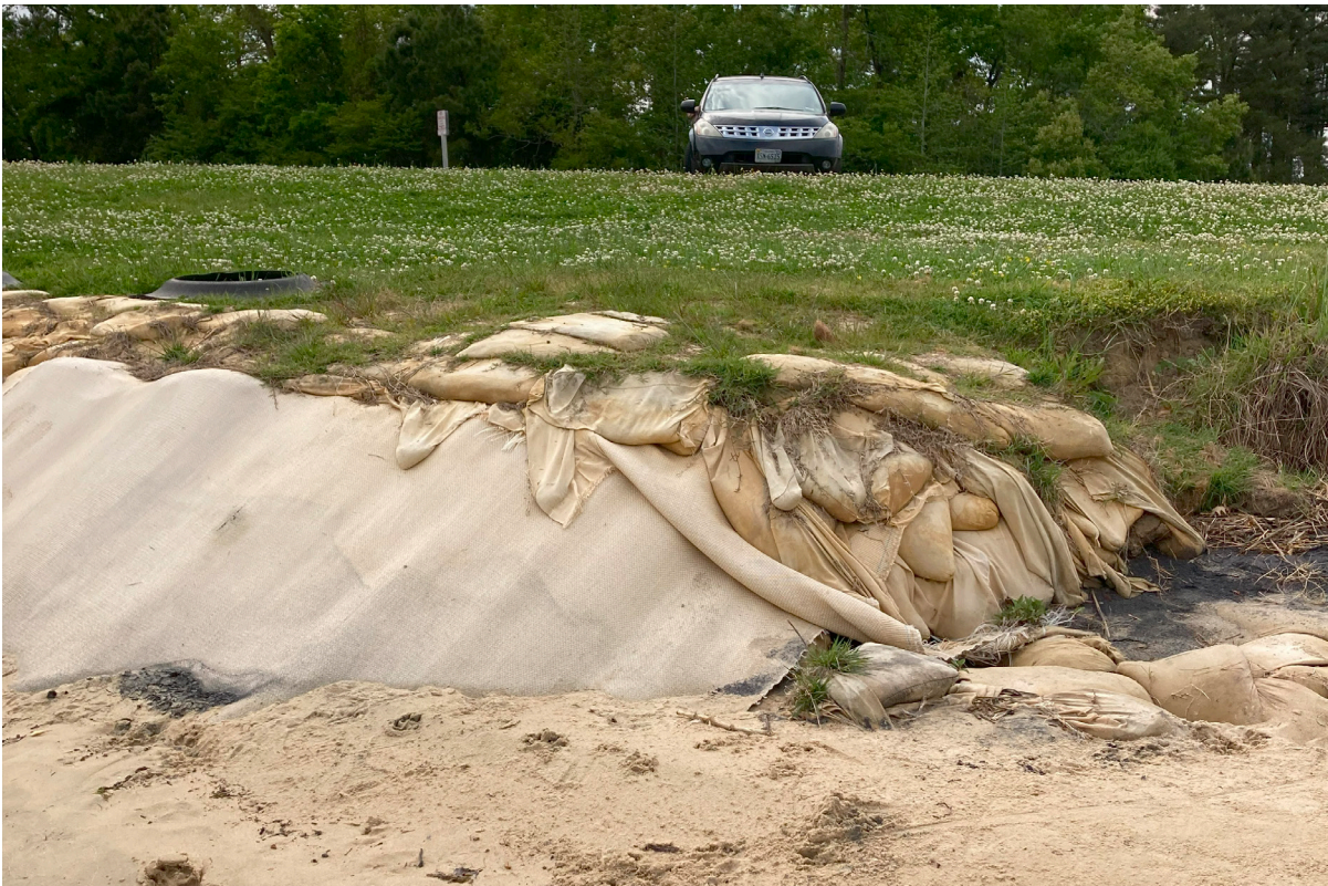
Figure 36. Eroding beach at existing parking area
